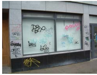
Defaced window and doors
