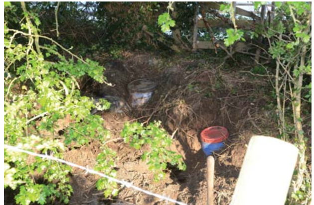
"Arms Dump" pipe buried in ground.
